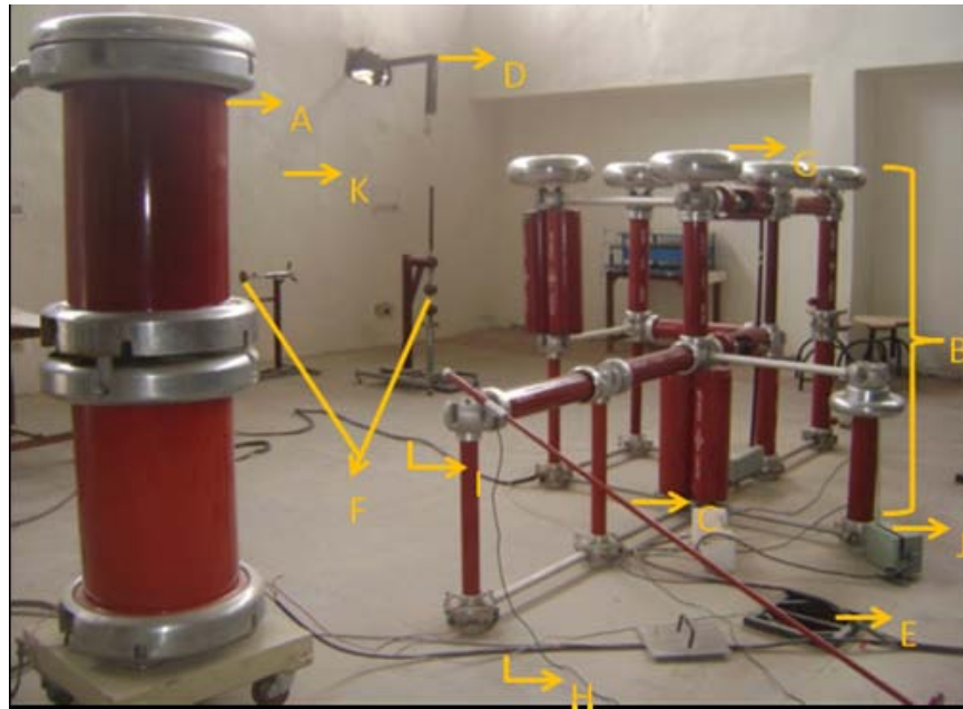
Fig. 1: Complete setup of HV equipment installed in NI-Hamirpur HVE laboratory
